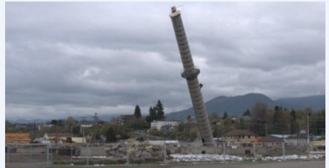
The mill site smokestack being pulled down after other attempts at demolition were unsuccessful
